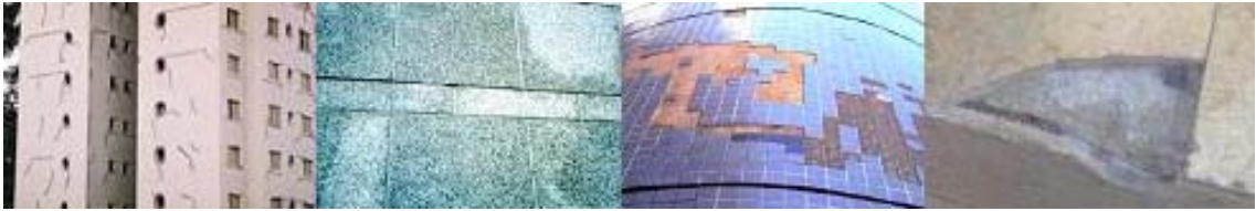
Figure 2 Different types of materials applied as façade coatings presenting anomalies
